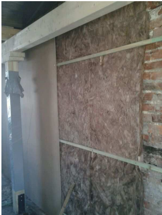
Figure 23: Internal insulation of the facilities chamber
